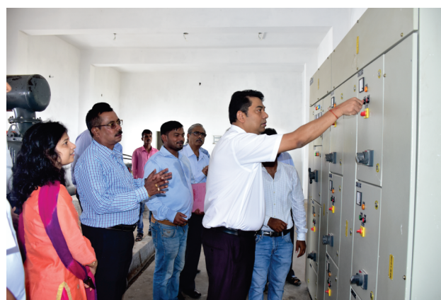
Paradip Port Chairman at the port's sewage treatment facility
