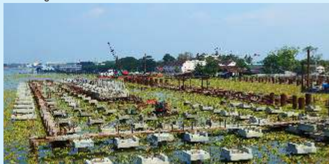
ISRF being Developed at CSL
