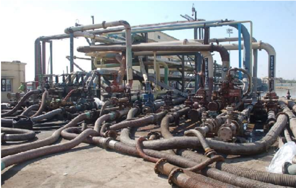
Figure 3-2 Cluster of Pipelines with Headers & Hoses
