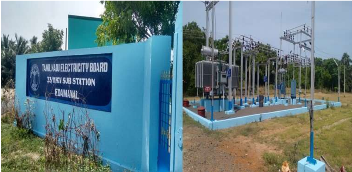
Figure 3.13 Electrical Substation at Edamanal
