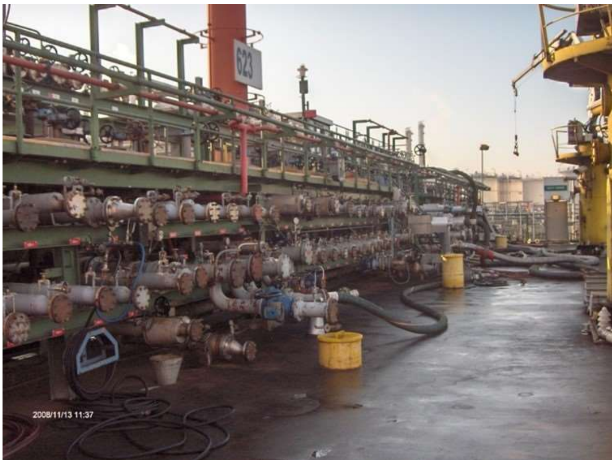
Figure 6-1 A Typical Jetty Head with Pipeline Headers at Antwerp Port
