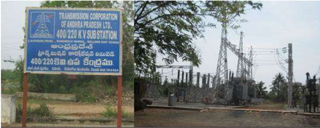
Figure 2.14 Electrical Substation near Manubolu
